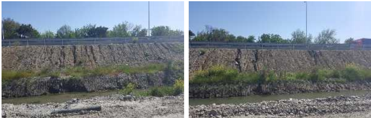
Figures 1 and 2: Erosion of slopes of embankment
