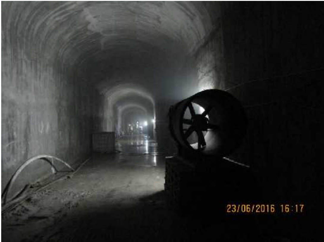
Photograph 5. Fans off when the tunnel is dusty
