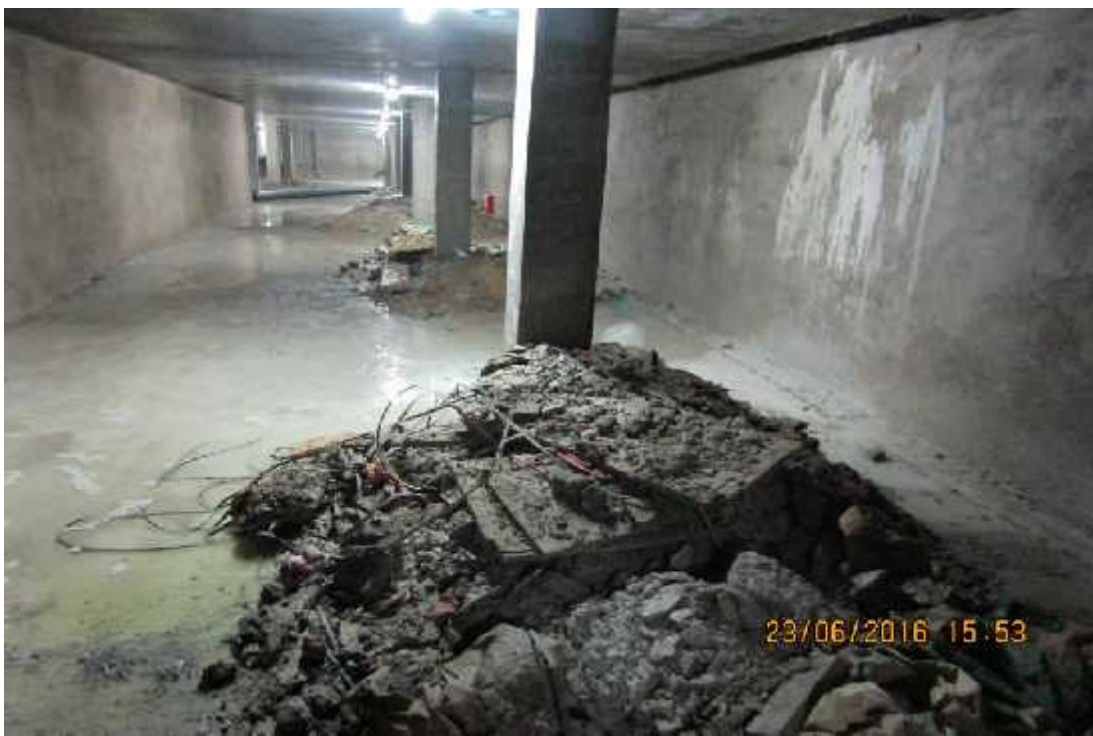
Photograph 6. Waste disposal inside the tunne
