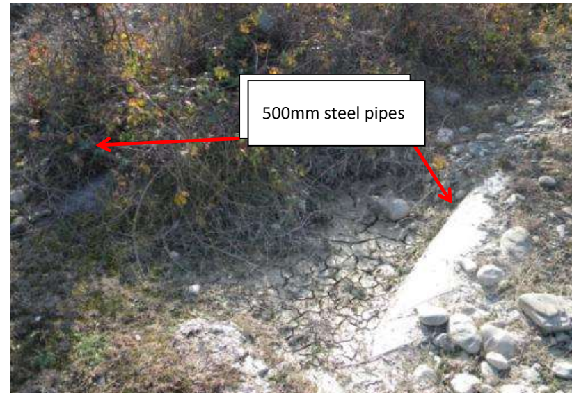
Site 4 - Ø 500mm steel pipes
