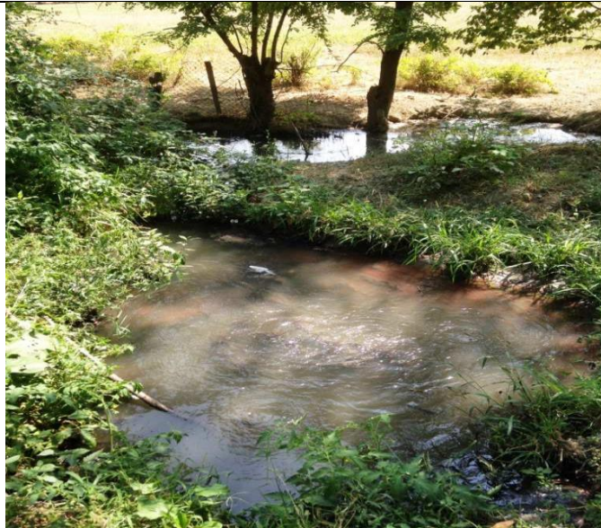
End of the old sewer trunk to Telavi WWTP beside the state road to Alazani Bridge
