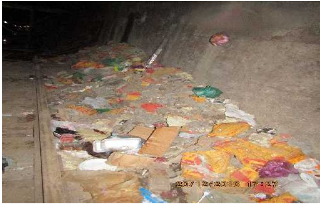
Photo 3: General Waste disposal inside the tunnel. The non-compliance has not been close
