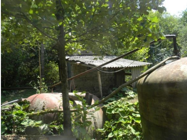
Area of the reservoir and pump station with chlorination unit
