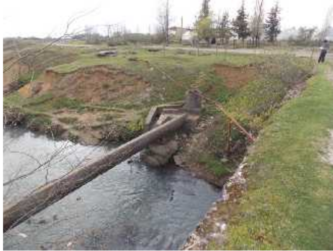
Picture 4.2.2. Untreated Wastewater Discharge Point
