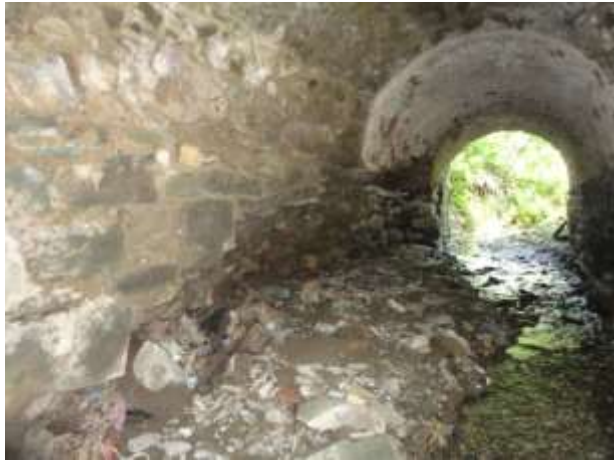
Ruined wall, view from exit
